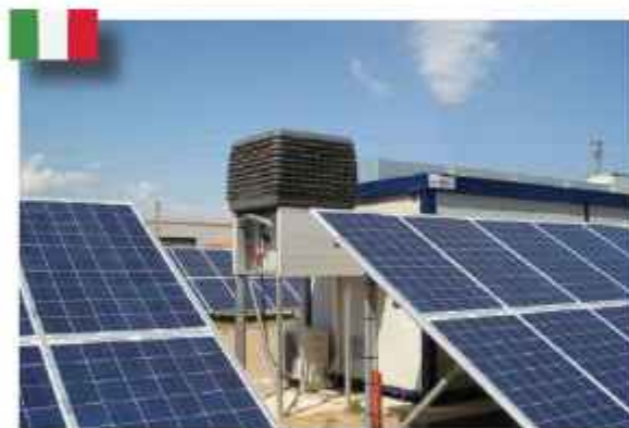
Solar panels Italy | SOLAR PANELS
